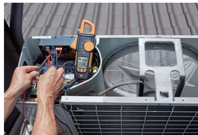
测量空调外机电压
